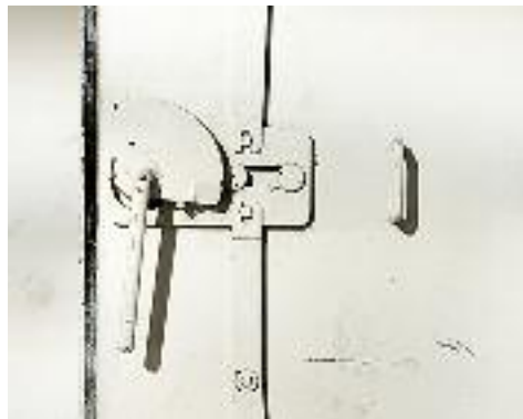
Habima Tiefgarage, Stadtzentrum Tel Aviv Habima underground parking garage, Downtown Tel Aviv
